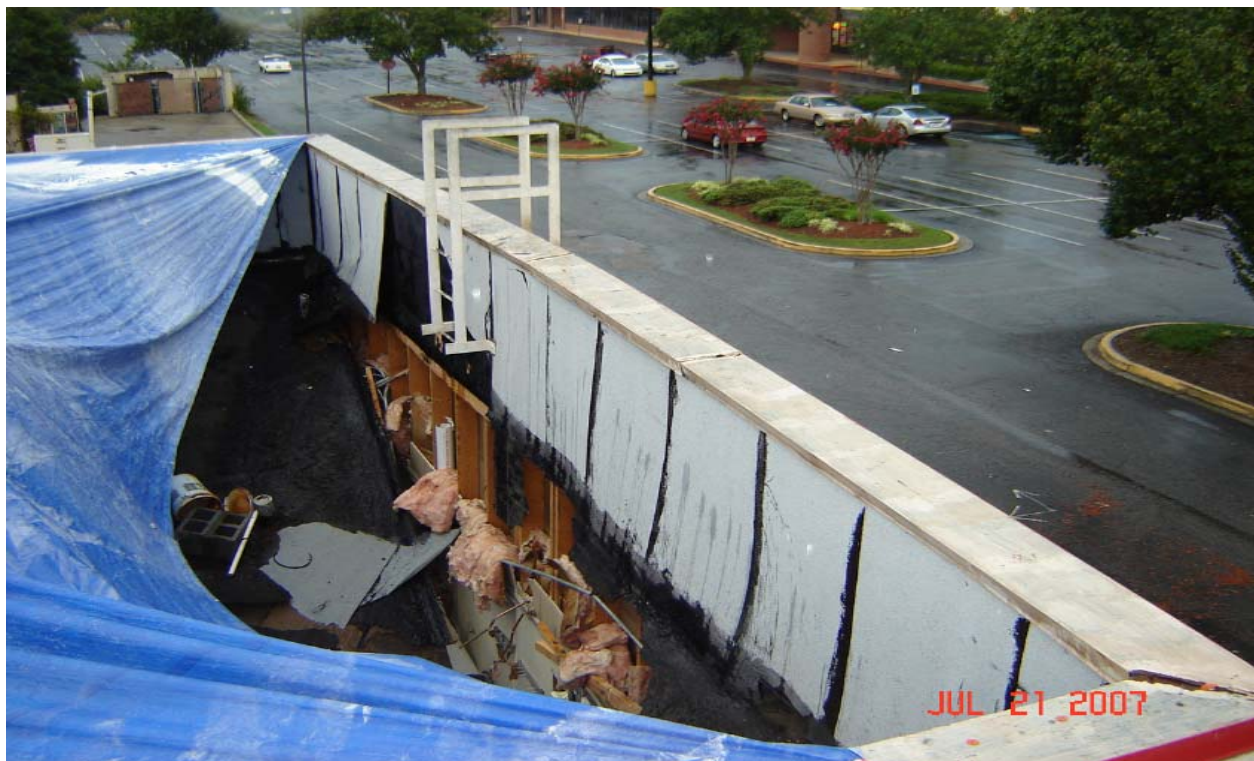
2. Collapsed roof over kitchen area
