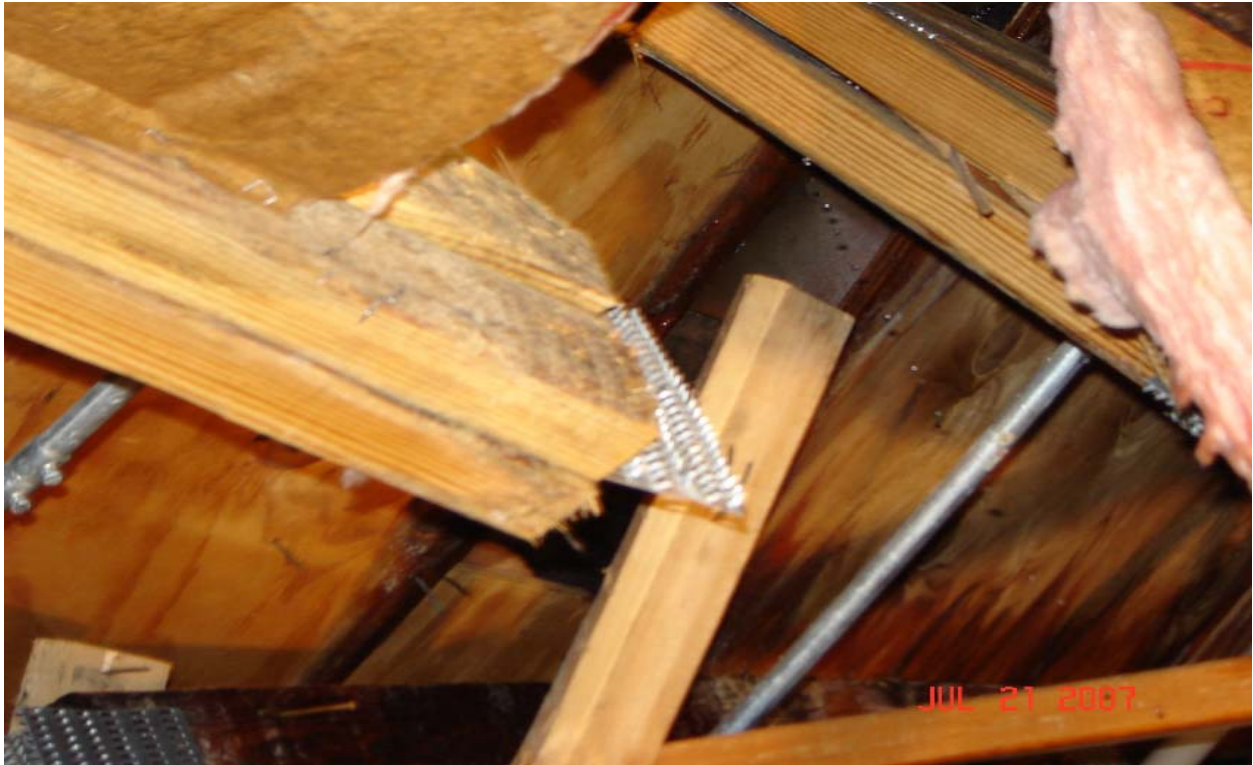
3. Broken trusses in kitchen area
