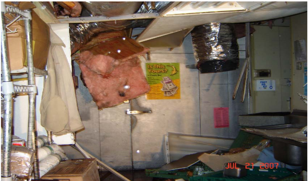
4. Damage in kitchen area
